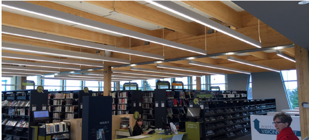
Via 2 pendant cable direct/indirect
